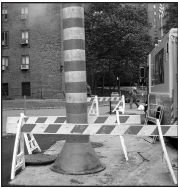
Photo #3--Vent stacks direct steam up and away from the roadway.
