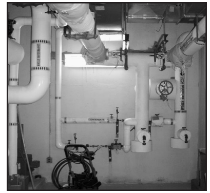
Photo #6--Steam room in a building supplied by Con Ed.
