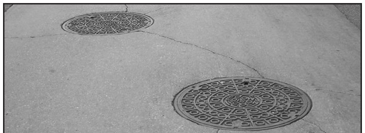
Photo #2--Steam manholes often are found in pairs, inserted into a concrete vault cover.
